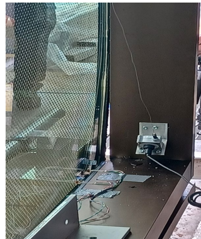
2. Damage state: detachment of glazing
